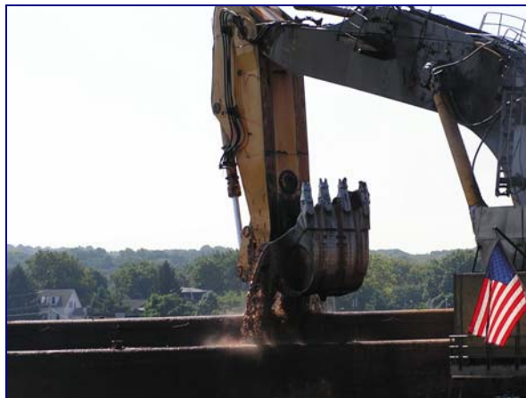
Bean Excavation, LLC dredge Tauracavor working at IMTT Pier A removing glacial till material for placement at HARS.
